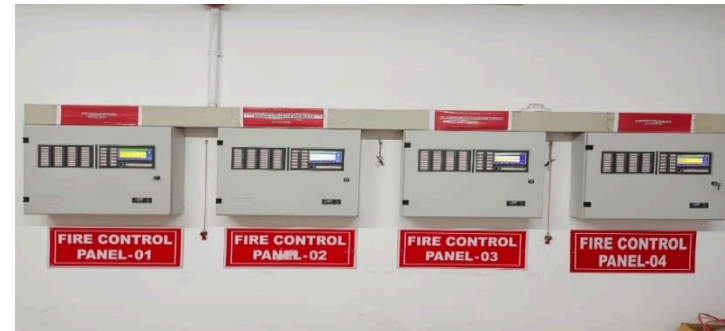
Addressable Fire Alarm Systems
